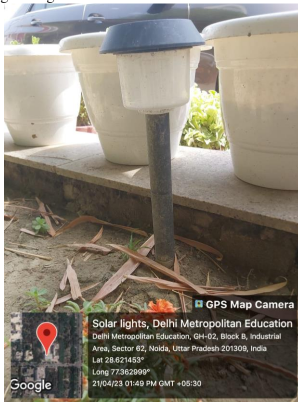
Solar Light in Garden
